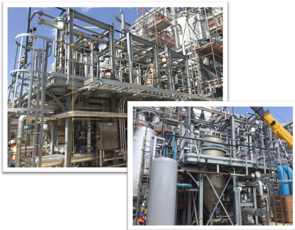
Figure 9: BHS Candle Filter Grey Water Installation
