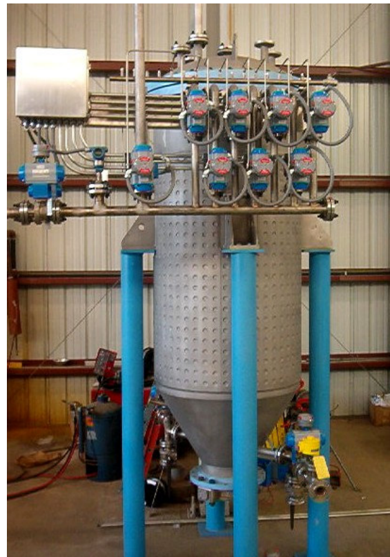
Figure 6: Jacketed Candle Filter with Register-Filtrate Piping & Junction Box
